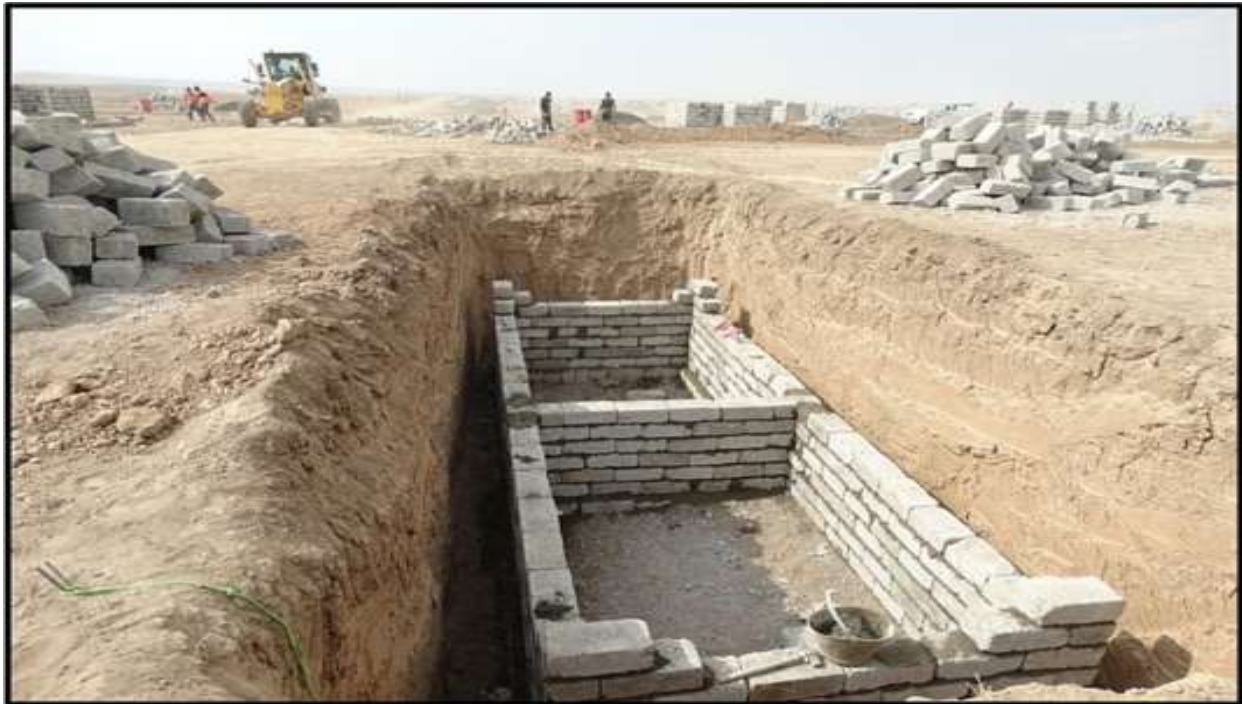
Figure 2: Blackwater containment for Kabarto 2 [6]
